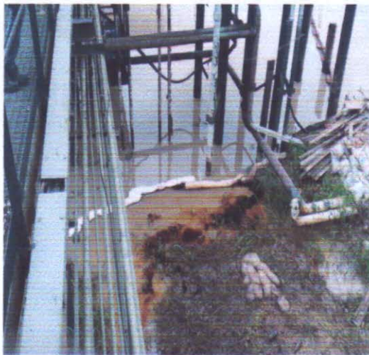
Fig C: picture showing failed boom
